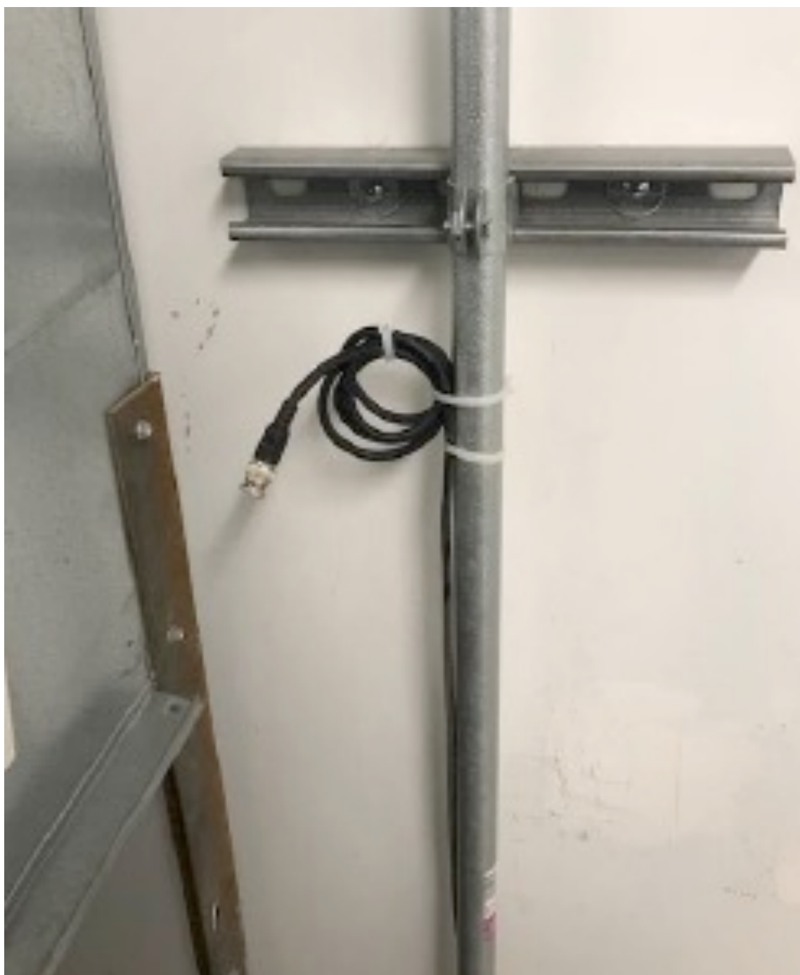
Coax Cable inside 3 rd FL Fan Room
